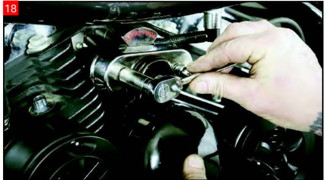
18 Use the included acorn nuts and washers on the studs of the vibration isolators. With a 1/2" deep well socket, tighten down the hardware.
